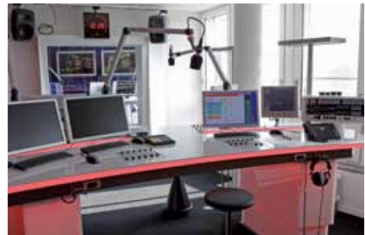
OnAir 2500 Modulo system installed at Studio 105, Zurich
